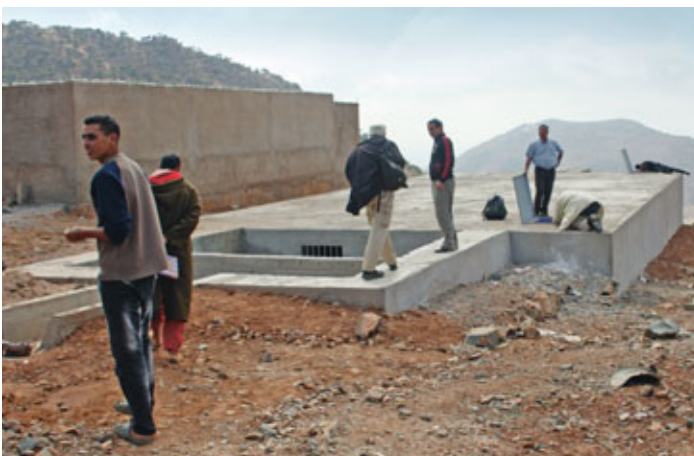
A large new cistern has been built on Mount Boutmezguida. It is located near the village school and stores water from the fog nets. This allows the villages in the valley to be supplied with water for several months.
