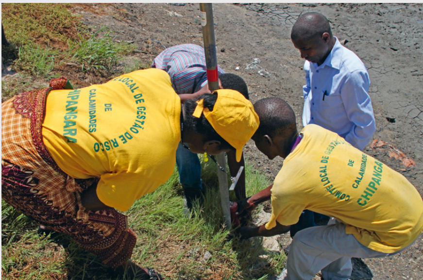
A key moment: representatives of the flood committee install a flood warning pole at a canal in Chipangara. Usually, there is no water in the canal for many months. However, in the case of strong rainfall it can become a hazard within a matter of hours and lead to flooding.
