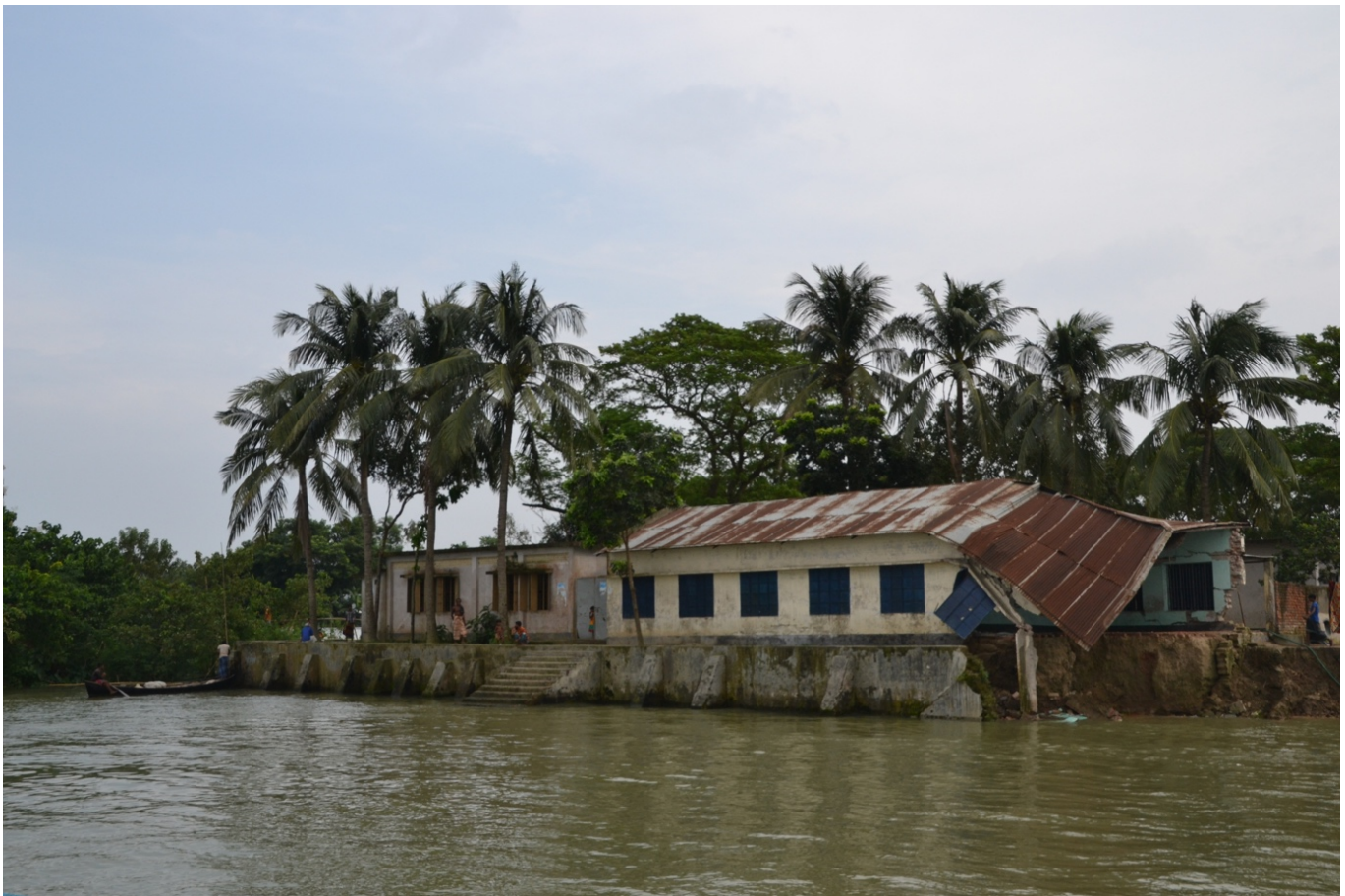
The riverbank erosion finally pulled half of the school building into the water (© Sonja Ayeb-Karlsson).
